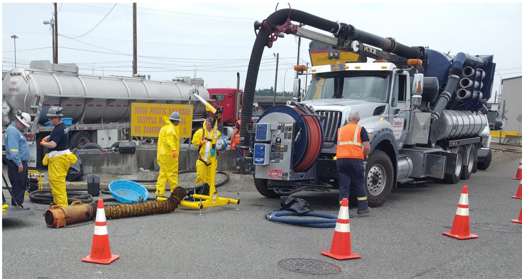
FIGURE 4: RESPONSE TO PCB SPILL INTO THE STORMWATER SYSTEM (PHOTO CREDIT: CITY OF SEATTLE)
